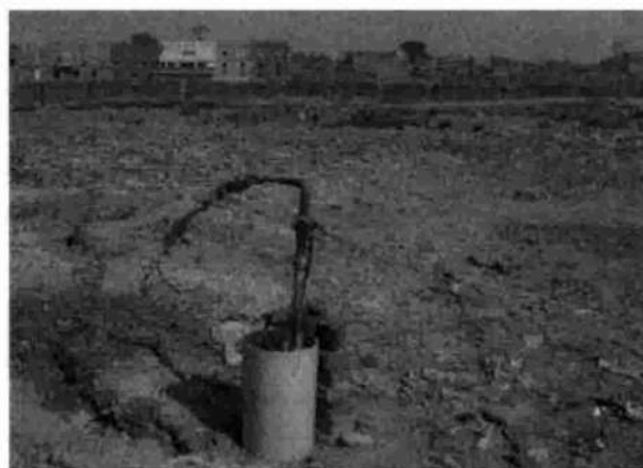
Step vi: Drawing water samples by installation of submersible pump in constructed well
